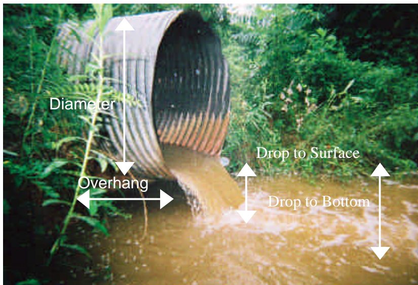
Figure 2. A typical pipe culvert with a drop to the tailwater surface (Camp Creek, Lumpkin County).
